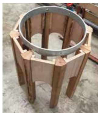
The original steel ring was re-used in the re-construction of the lantern.
