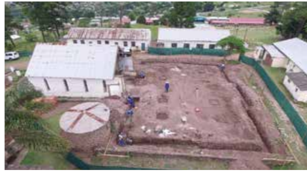
Drone photograph showing the original nave retained and the trenches for the extension.
