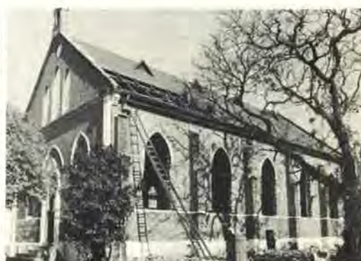
NEW SCOTLAND CHURCH, CNR LOOP AND BUCHANAN STREETS In course of demolition - site now a parking lot
